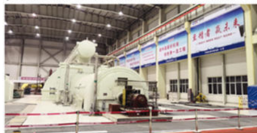
1. Caofeidian was the first plant in China to incorporate three low-pressure casings in the steam turbine. Courtesy: Shanghai Shenergy Power Technology Co. Ltd.
